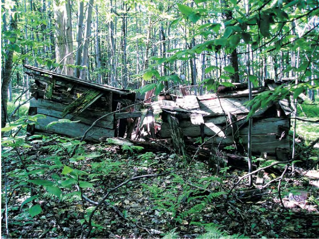
Photograph 27. Collapsed log structure at the Saphouse Site (OPRHP Site 01907.000086); view to the southwest.
