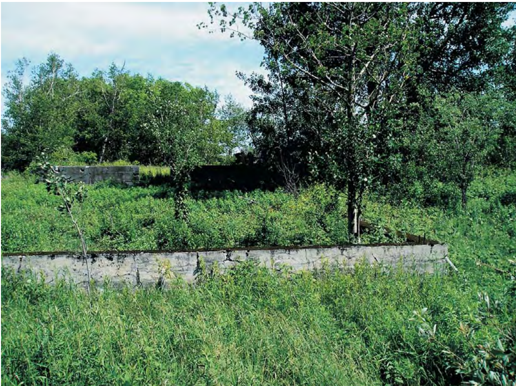
Photograph 20. Cement foundation remains of the mill works at Clinton Mills (OPRHP Site 01907.000088); view to the east.
