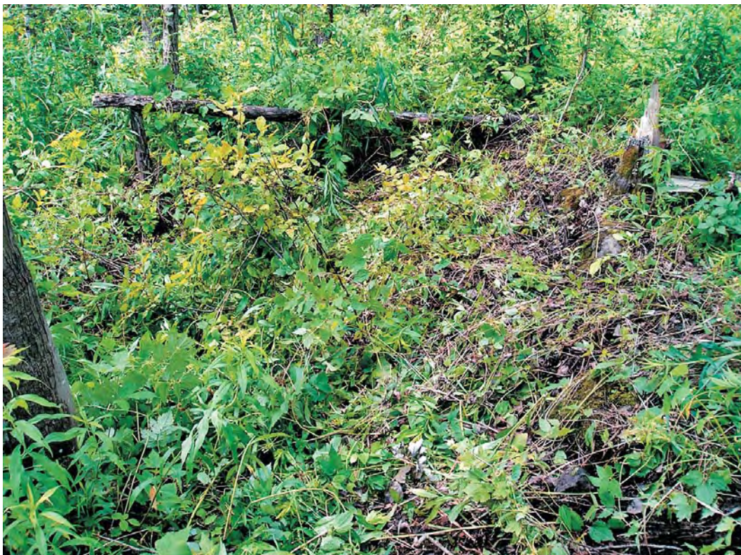
Photograph 28. Overgrown and pushed-in foundation at the Boomhower & Humphrey Site (OPRHP Site 01907.000082); view to the north.
