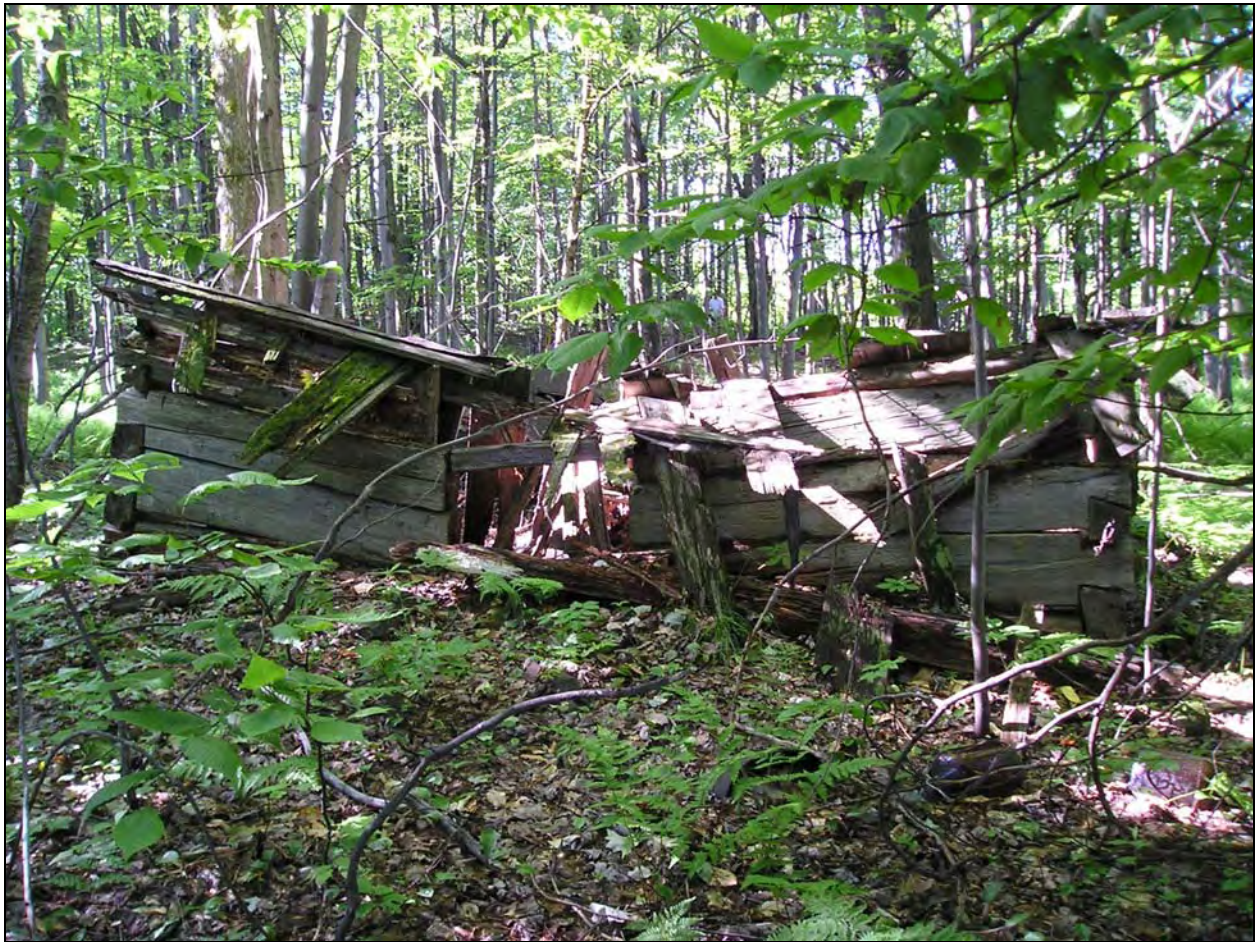
Collapsed log structure at the Saphouse Historic Site (view to the southwest).
